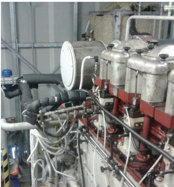
Fig. 2 Diesel generator (diesel-generator unit (DGU) - 900) with soybean oil supply system as fuel
